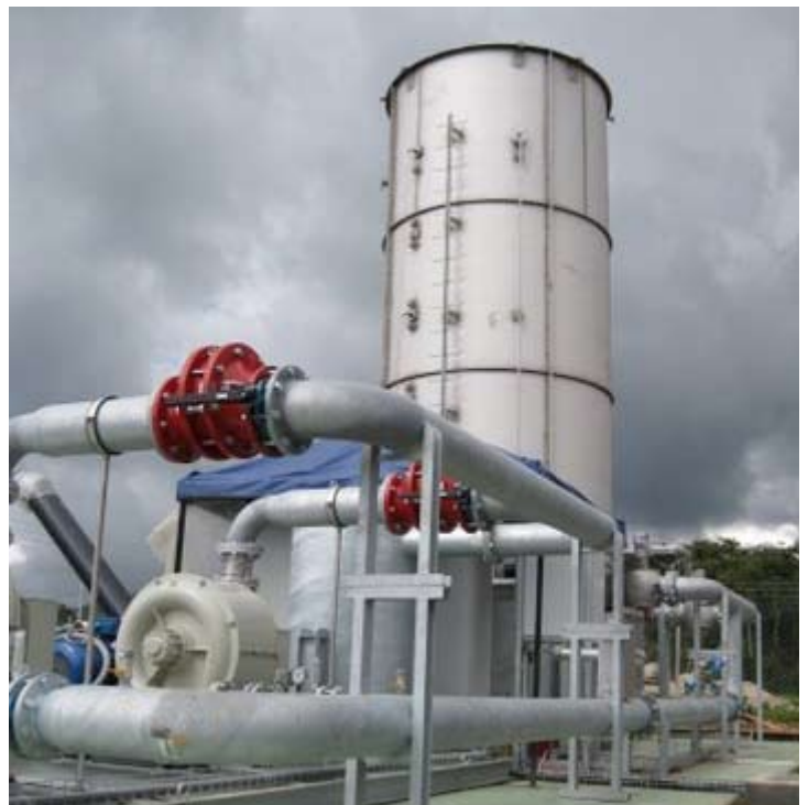
The flare unit ready to start operating
