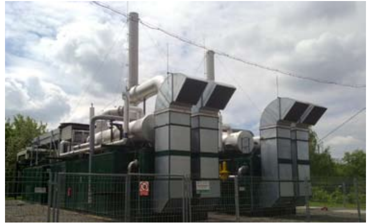
The 22nd CHP unit installed by Green Gas DPB
